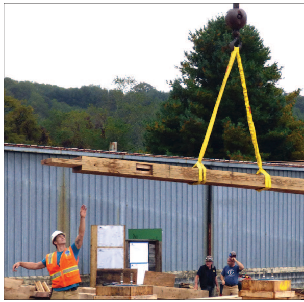
Guided by a guild member, a crane moves a beam into place.
