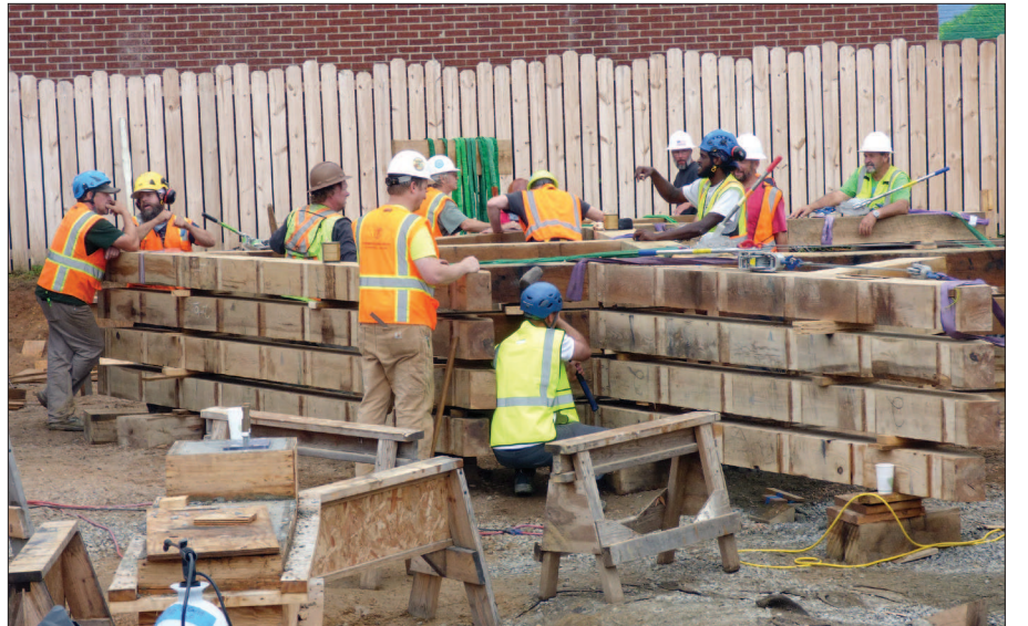
Workers prepare the wooden cross-sections of the structure, called bents, which will be lifted by a crane and set in place.
