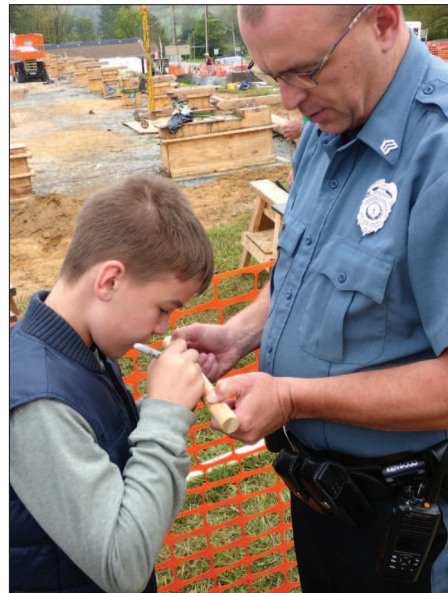
Cooper Adams (left, with father Matthew Adams) signs a wooden dowel, which workers later hammered into place. There are many hidden items inside the structure, including a 2021 quarter.
